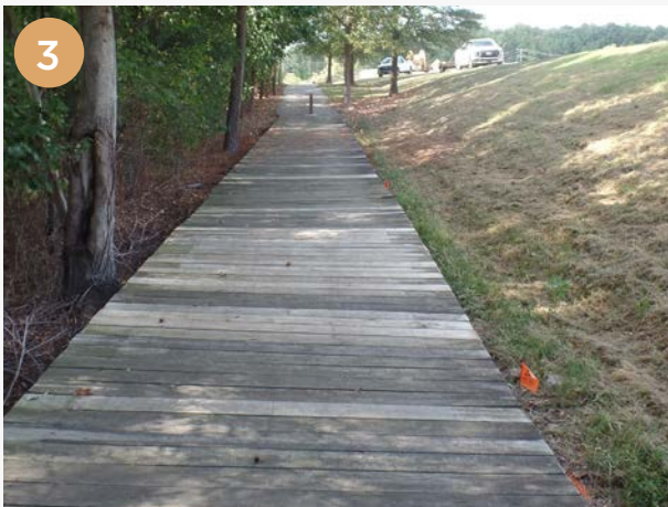
Bridge Location: Park Center Loop Trail, west of the Research Triangle High School driveway. Dimensions: W - 8', L - 180', H - 0" Key Notes: - Some mold/mildew growth noted, older bridge, no railings; bollards located at bridge entrance, should be painted brighter color for visibility Recommendation: Remove mold/mildew and apply paint with a grit substance to improve traction. Paint bollards a brighter color for visibility.
