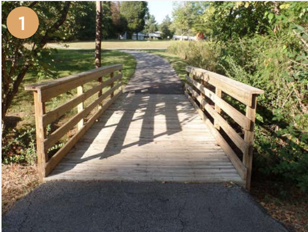
Bridge Location: Park Center Loop Trail, south of Maughan Dr. Dimensions: W - 8', L - 25', H - 45" Key Notes: - Decent bridge condition - Trail approaches bridge at an angle Recommendation: Apply paint with a grit substance to improve traction.
