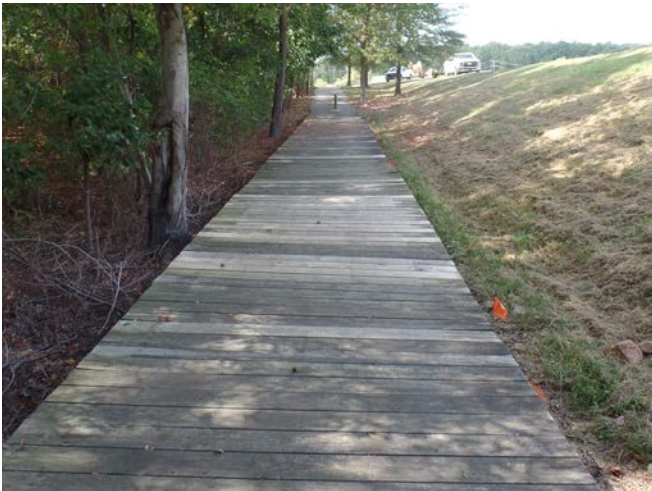
Above: Boardwalk example that avoids issues with roots from adjacent trees (NC 54 near Research Triangle High School)
