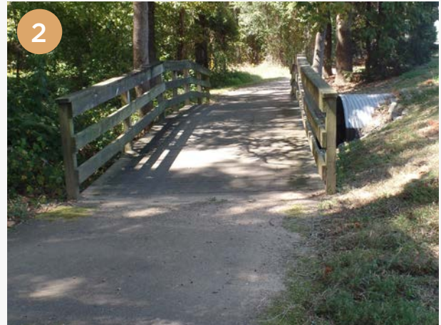
Bridge Location: Spur Trail (NC 54), west of TW Alexander Dr. Dimensions: W - 8', L - 36', H - 36" Key Notes: - Some mold/mildew growth noted, older bridge Recommendation: Remove mold/mildew and apply paint with a grit substance to improve traction.
