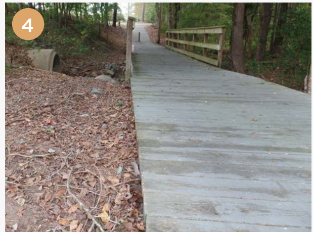
Bridge Location: Park Center Loop Trail, east of the Progress Center driveway. Dimensions: W - 8', L - 85', H - 45" Key Notes: - Some mold/mildew growth noted, older bridge; bollards located at bridge entrance, should be painted brighter color for visibility Recommendation: Remove mold/mildew and apply paint with a grit substance to improve traction. Paint bollards a brighter color for visibility.
